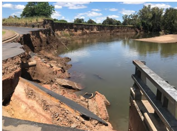
Photograph 5. Resultant damage to the reserve and approach to the southern end of the Duke of Wellington Bridge
